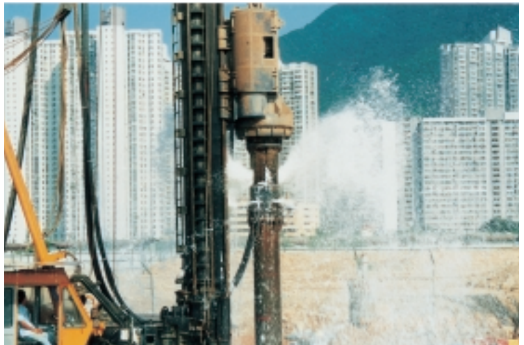
Foundation Foundational construction of buildings and bridges up to 32''(Ø800) of casing diameter.
