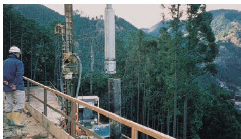
Piling After casing through the collapsing overburden, insert a H-steel, then pull up the casing.
